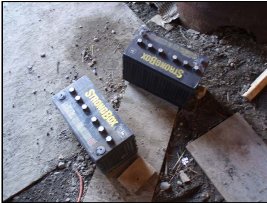
Photograph 19: Lead-acid batteries observed in the City Shop.
