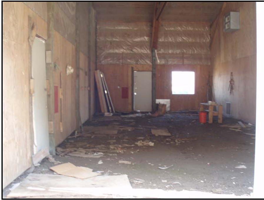
Photograph 15: Inside Section 1 of the City Shop (northern most portion). This section had been cleaned out by the City prior to the site visit.
